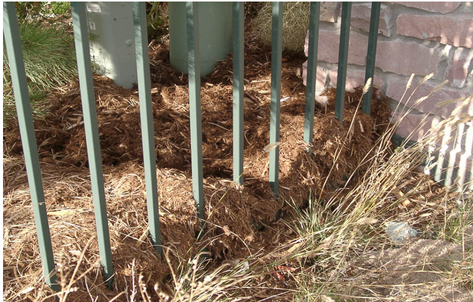
Wood mulch installed too thick is gathering above grade along the view fence. This is not permitted.
