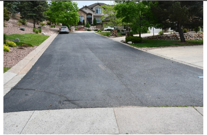
Photo #29 – Pavement – Glen Arbor
